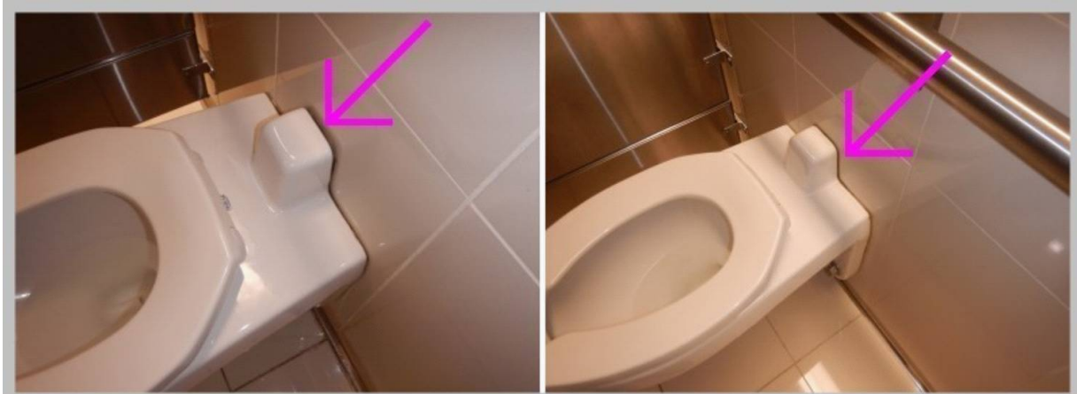
Men's & Women's loose & lack caulking
